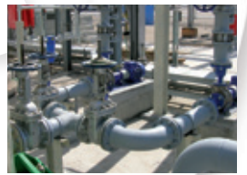
M U.A.E., Ruwais Petrochemical production plant
